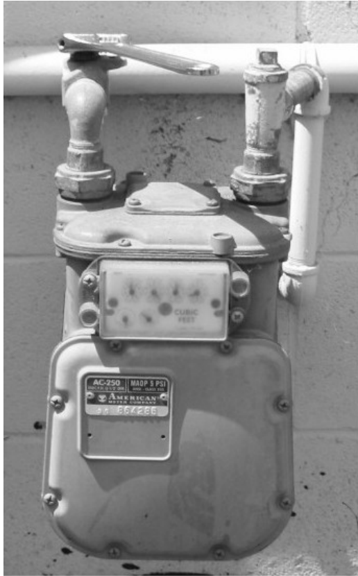
Photo illustrating a natural gas meter with an adjustable wrench on the ¼ turn shut off valve
